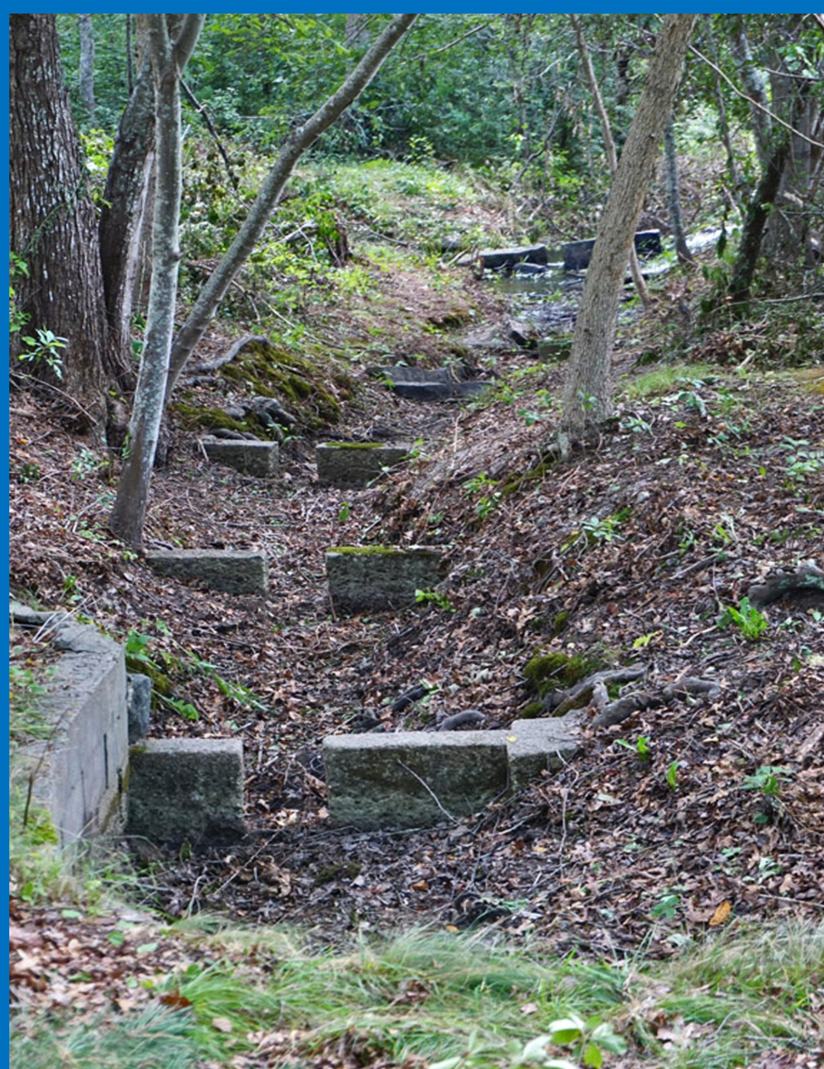
August 2020 Non-functional Fish Ladder
