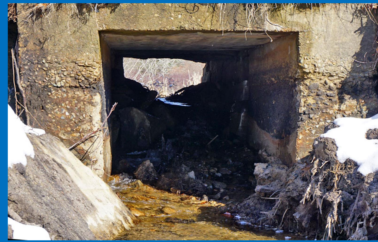
Early February 2021 – Deteriorated Culvert
