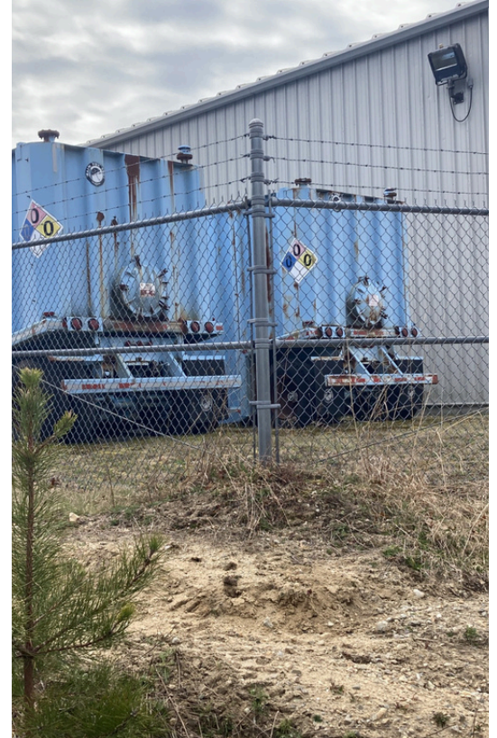
Look for this pumping station while you are walking the trail!
